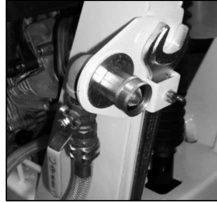
Figure 17: Water Supply Fitting
